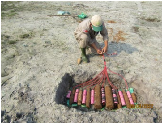
A PeaceTrees EOD technician preparing for an on-site demolition of explosives-Quảng Trị Province
