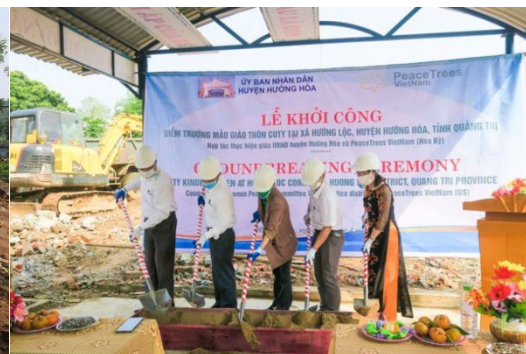
PeaceTrees staff and partners break ground on the Cu Ty Kindergarten project- Quảng Trị Province
