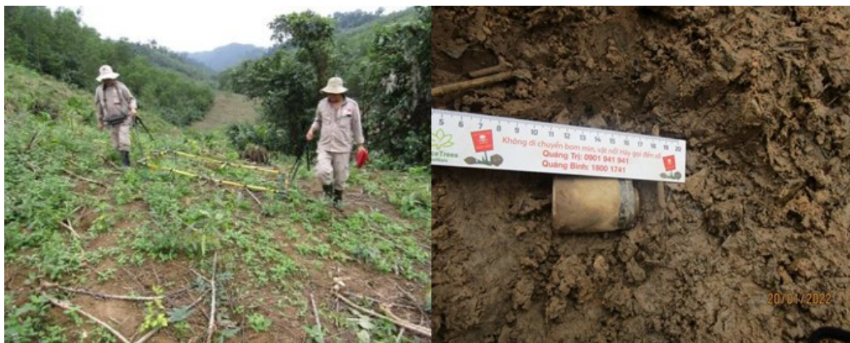
A pair of PeaceTrees EO technicians working to clear the future banana site in Ta Lao Village
