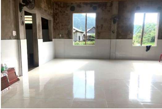
An inside look of the construction progress at the Cup Kindergarten- Quảng Trị Province
